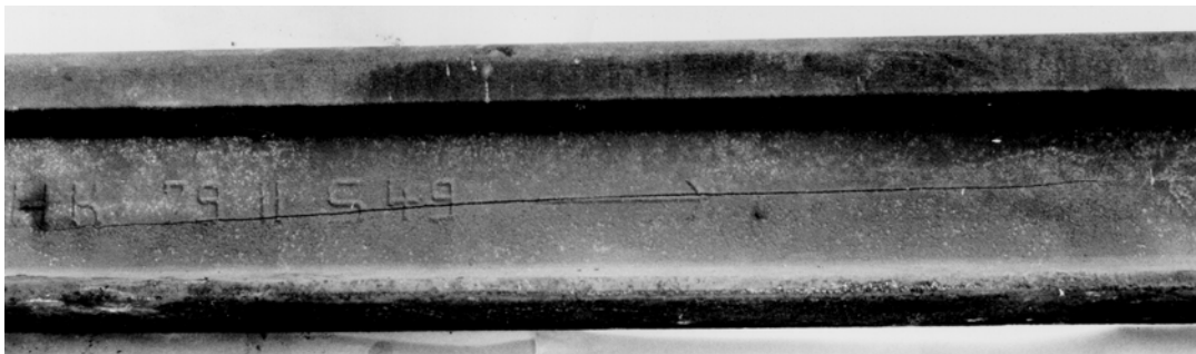
Figure 37: Horizontal web crack.
