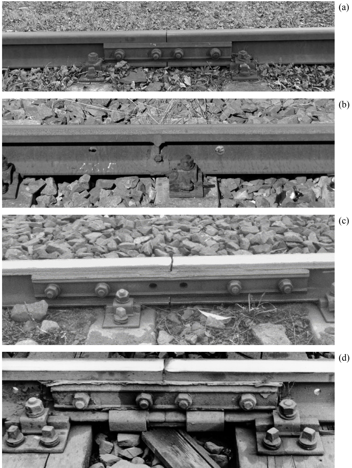
Figure 3: Rail joints. (a) fishplate with bolts; (b) continuous (aluminothermic) welded rail; (c) fishplate joint of a broken rail; (d) defective isolation joint.
